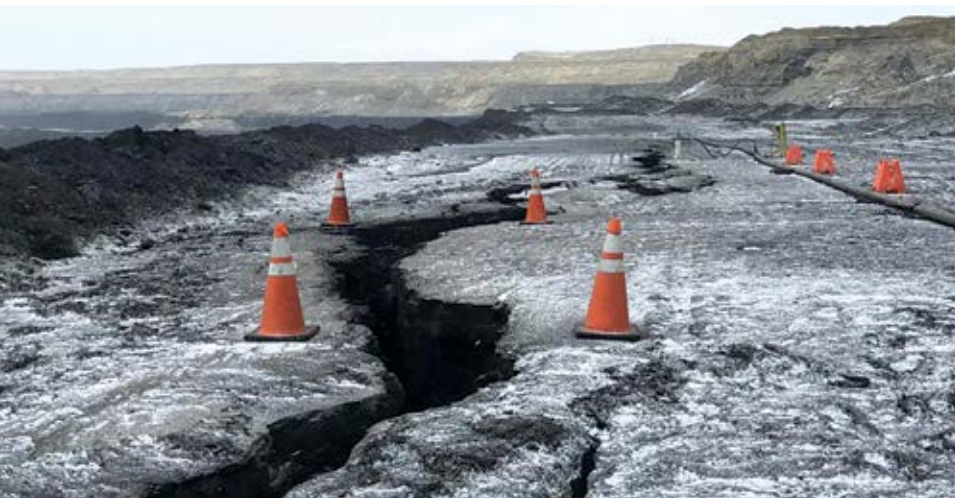
A 2-ft crack opened and widened along the coal seam dewatering structure at a mine in Wyoming. It prompted a special blasting project managed by a Blast Optimization Team, which used TITAN products to accomplish their goals. (Image: Dyno Nobel)
