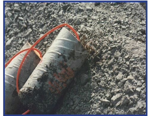
Figure 133 - Any booster tumbling in borehole is likely to break these shock tube leads.
